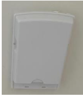
Fiber termination box (in closet 2 nd floor)
